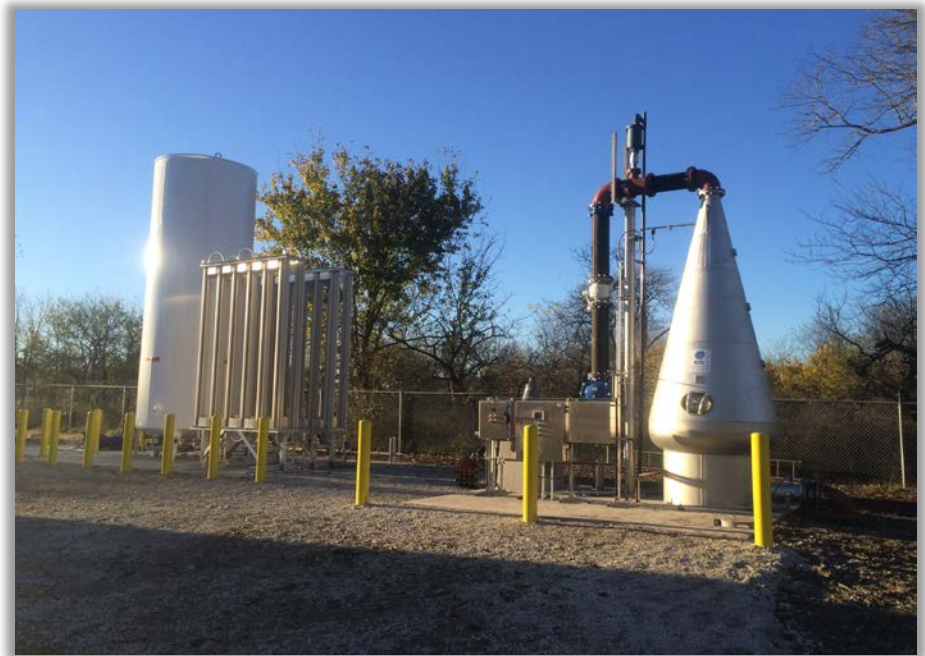
Installation of ECO 2 SuperOxygenation System at the Owen Good Pump Station, Raymore, MO
