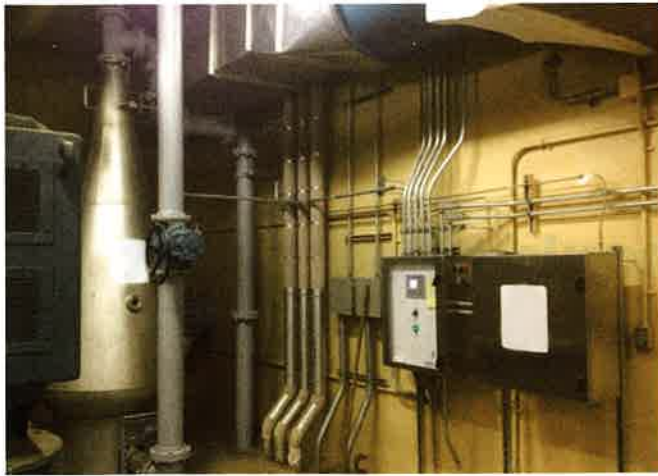
In addition to altering and automating the flow controls at the Gulf Pond Pump Station, Milford also added a sidestream treatment process to add pure oxygen to wastewater flowing through the force mains. This automated system helps ensure that the conditions inside the lines do not become septic. Charlie Smith/AECOM
