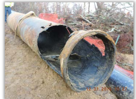
Sewer Pipe with H_2S Corrosion
