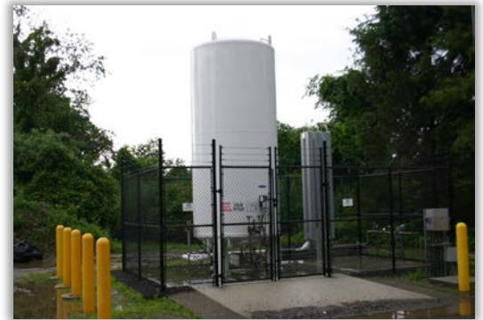
Bulk Oxygen Storage Tank
