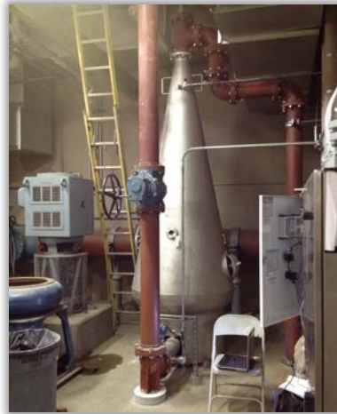
ECO 2 System Installed
