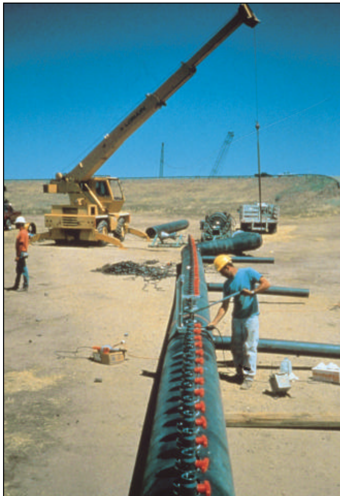
View of the 150-foot long diffuser used to distribute oxygen-rich water in the hypolimnion layer of the lake.
